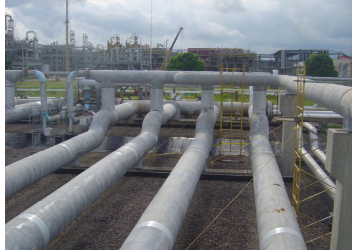
An overview of the "Slug Catchers" manifold.
